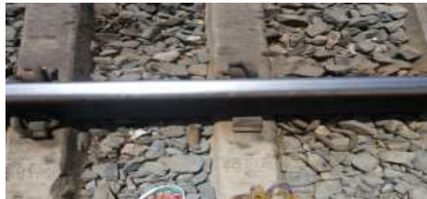
Fig no: 1.2 Broken Clamps in Railway Track
