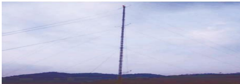
Figure: 3 Wind monitoring station installed at Rombagre, Meghalaya
