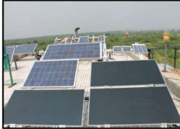
Fig.1 Solar PV System at Solar Lighting Laboratory Teri
